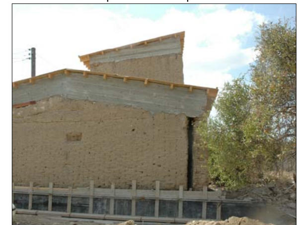
Incompatible concrete beams to support the roof & strengthen the foundation
