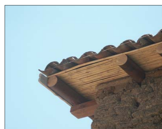
Construction of new roof (with tiles & cane) on a mud brick wall
