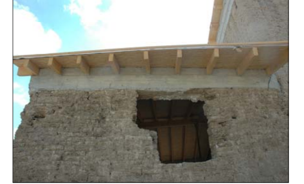
Non compatible concrete beam
